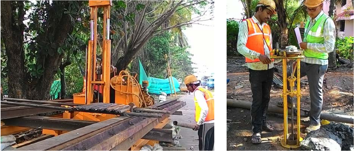
Fig. 2: Field investigation in progress. Photograph on left shows dead load placed over the Static cone penetrometer rig since the anchors could not provide sufficient reaction. Photograph on right shows field vane shear test in progress
